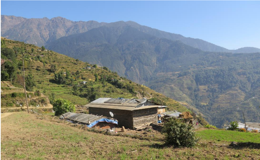
An earthquake resistant home being constructed in Bigu VDC, Dolakha district, November 2016. © Amnesty International
